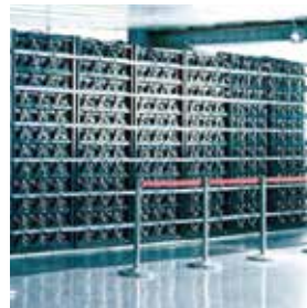
Energy storage system
