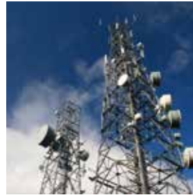
Communication power supply
